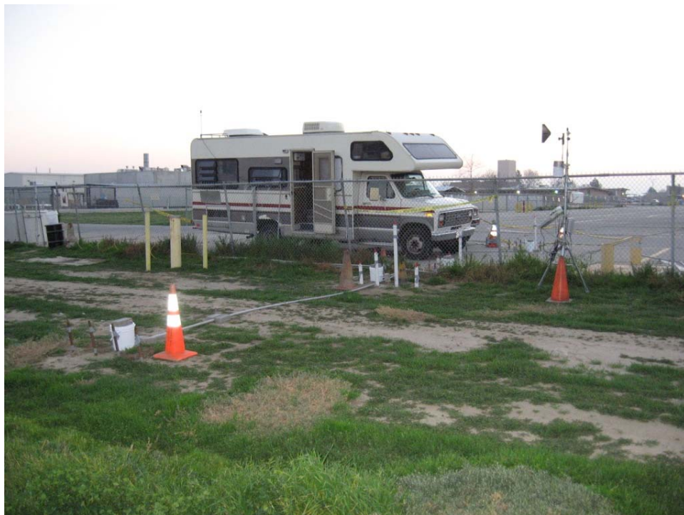
Photograph 18: Auto-sampler RV. Conduit running from probe locations to RV visible in middle ground.
